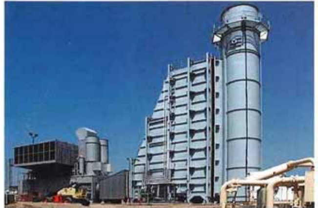
Burbank Water and Power Olive -voimalaitos.
